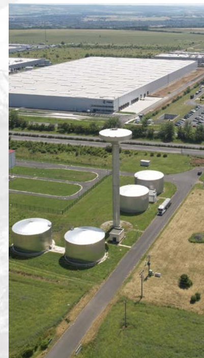
Water tower with drinking water and water tanks with filtered river water / vodovjem s pitnou vodou a zásobníky průmyslové vody
